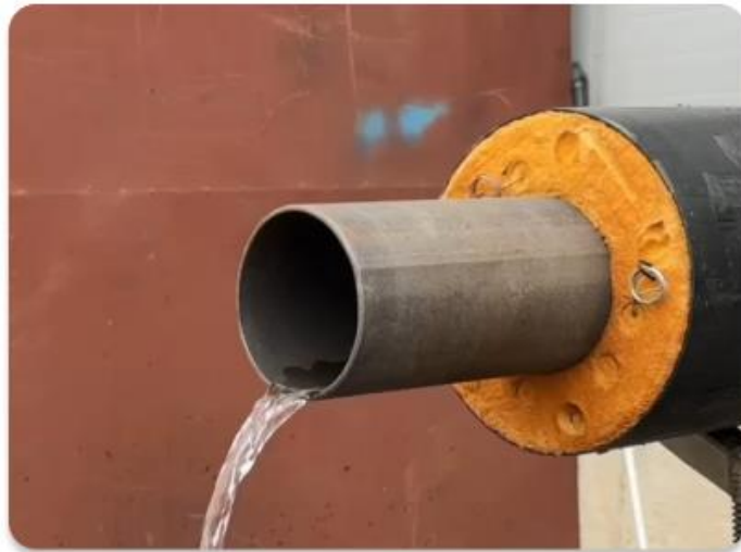
Commonly occurring water flow that impedes work.
